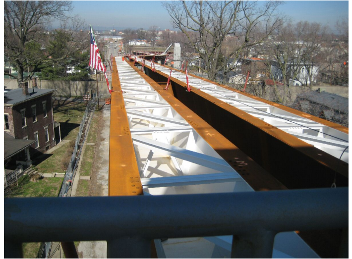
The support structure for the ramp in Jeffersonville, IN is in place. (photo courtesy Andy Murphy)
