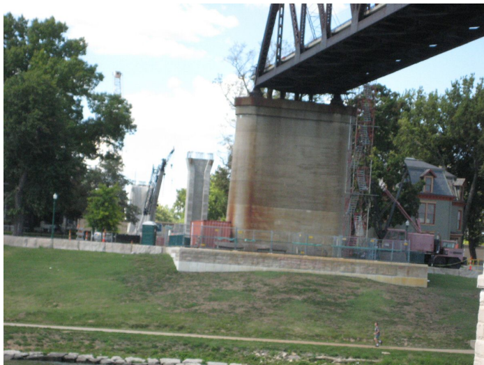
Support structure for Indiana ramp from the Big 4 Bridge is in place. (photo courtesy Andy Murphy)
