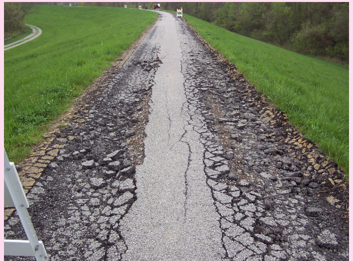
The damage left behind. (credit Kevin Brooks)
